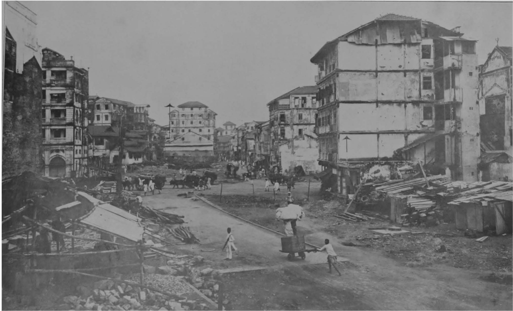
Sydenham Road under construction at its crossing with Masjid Bunder Road looking South; arrows indicate final breadth of Road.
