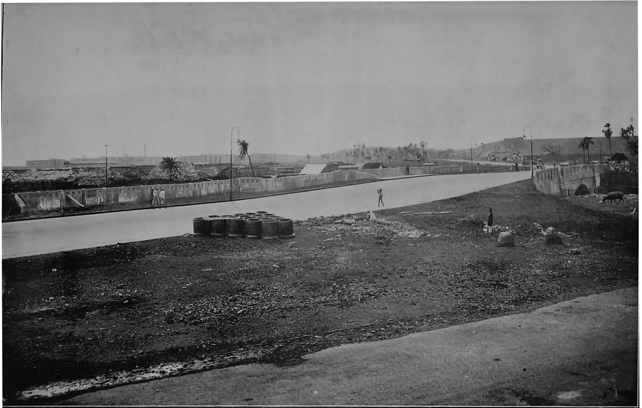
View of the New R. I. F. Bridge over Municipal Storm Water Channel along Road No. 5 (Worli Road) looking South and taken from W. W. Corner.
