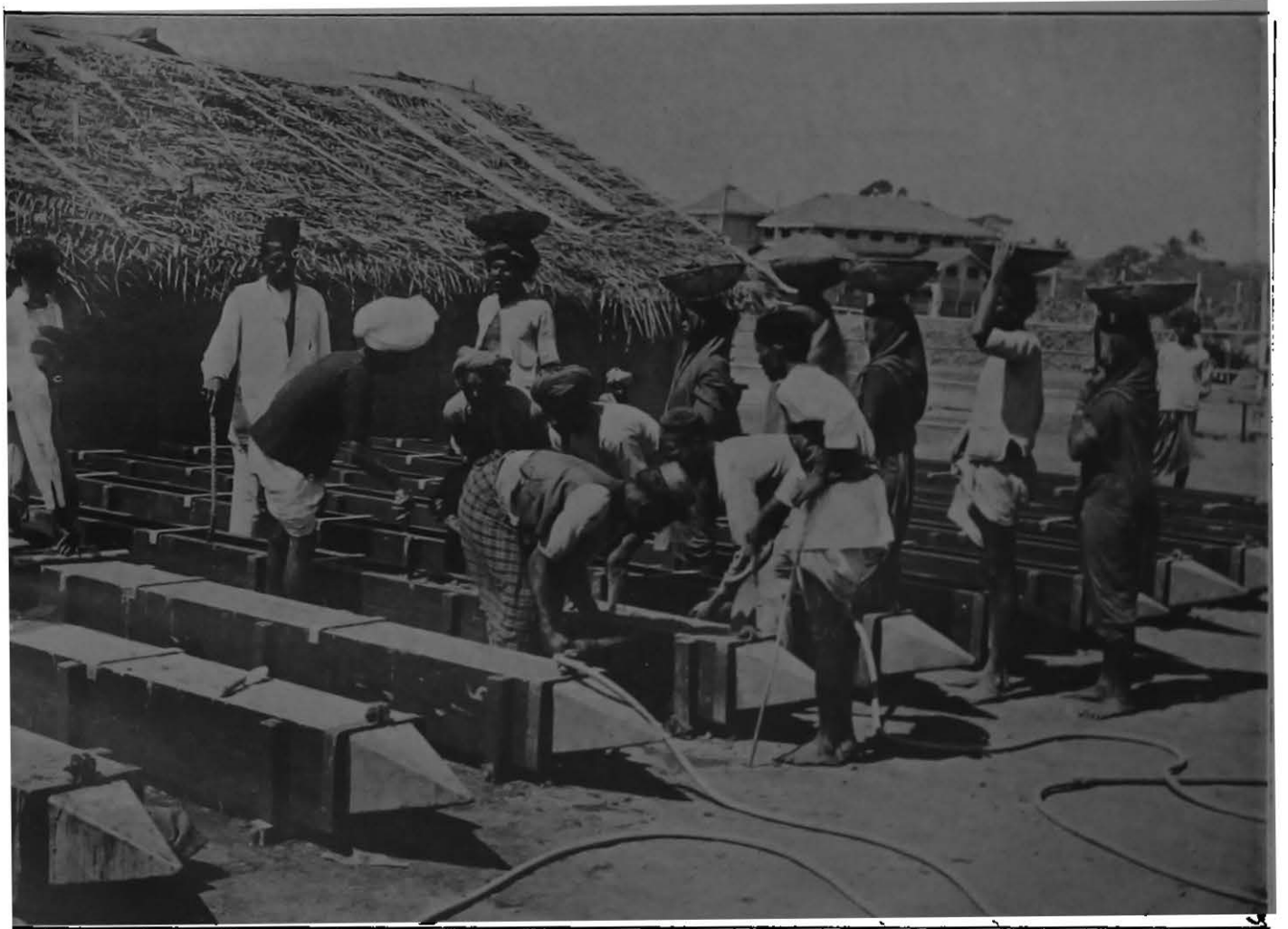
6—Kennedy Sea Face, Bombay—Filling reinforced cement concrete piles, showing method of vibrating the moulds with pneumatic hammers. 21st March 1915. Work commenced—20th February 1915. Number of piles completed upto 21st March 1915—77.
