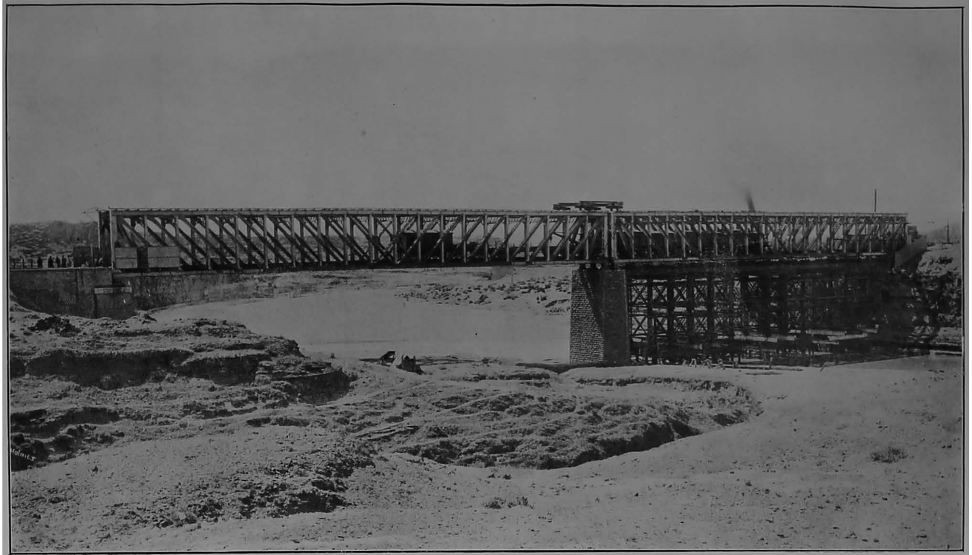
Strengthening of Haro Bridge, North Western Railway (in progress), to carry standard III loads.
