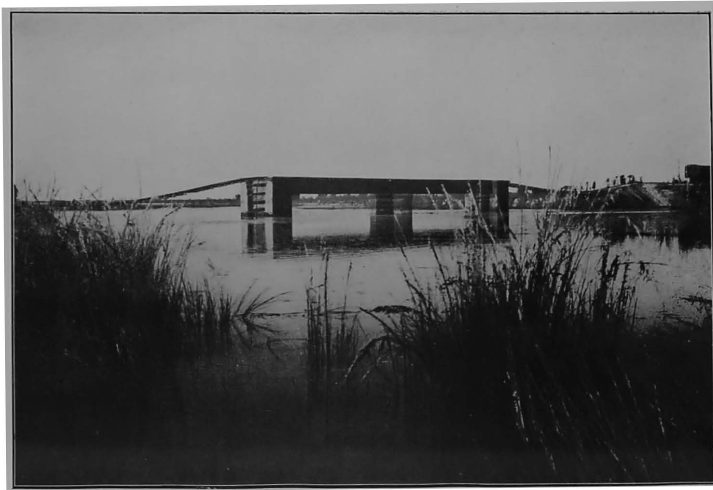
60' girder bridge at mile 480, main line, Oudh and Rohilkhand Railway, after the floods.
