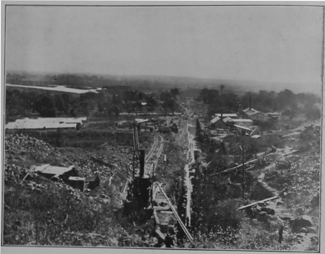
Parik tunnel, Great Indian Peninsula Railway, under construction, view from Eastern Portal.
