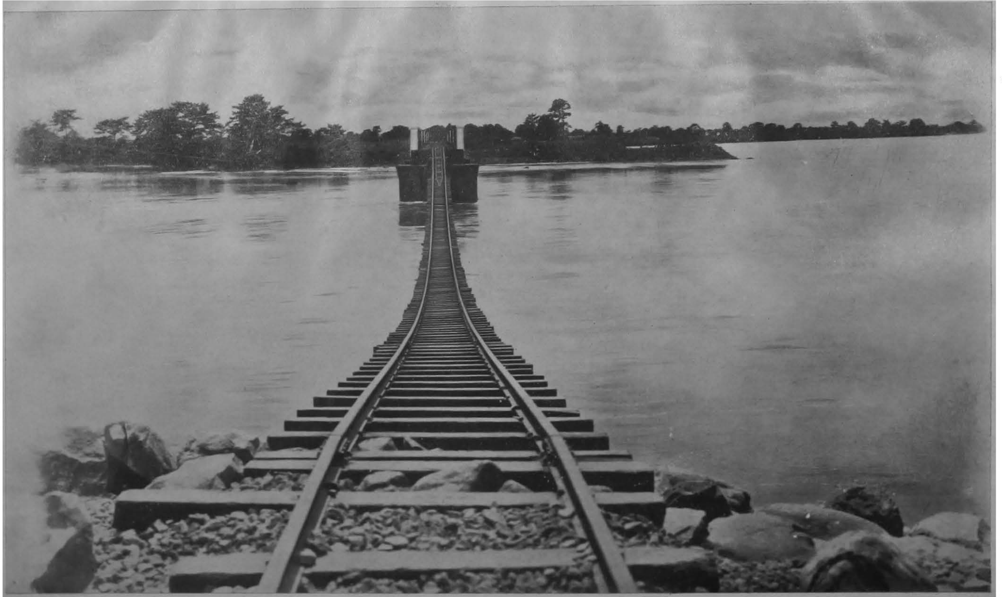
The effect of floods. Breach at Aie Bridge between Bongaigaon and Bijni.
