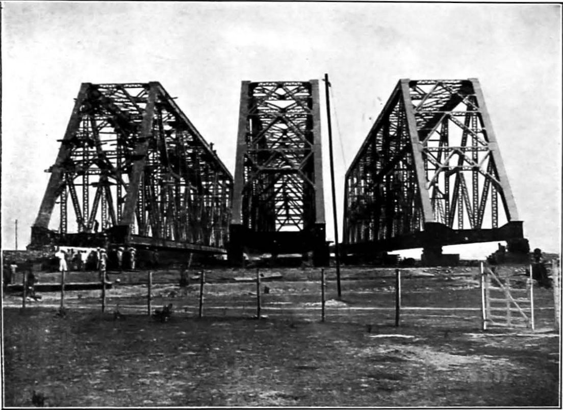
Three spans in the stacking yard ready for removal to bridge site.
