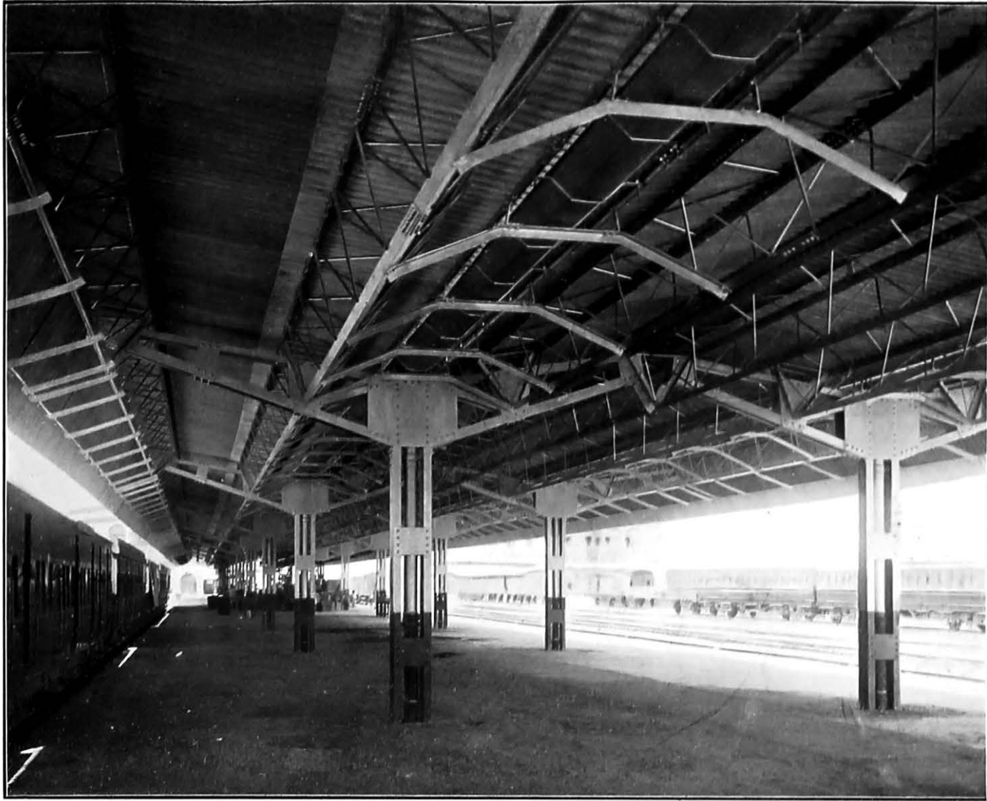
Platform passenger shelter at Karachi City station, showing the all-welded 50 feet long purlins of angles and round bars.
