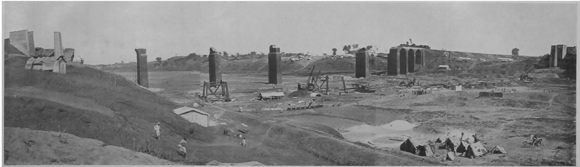
GENERAL VIEW SHEWING CONSTRUCTION OF THE NEW BRIDGE AND REMAINS OF THE OLD.
